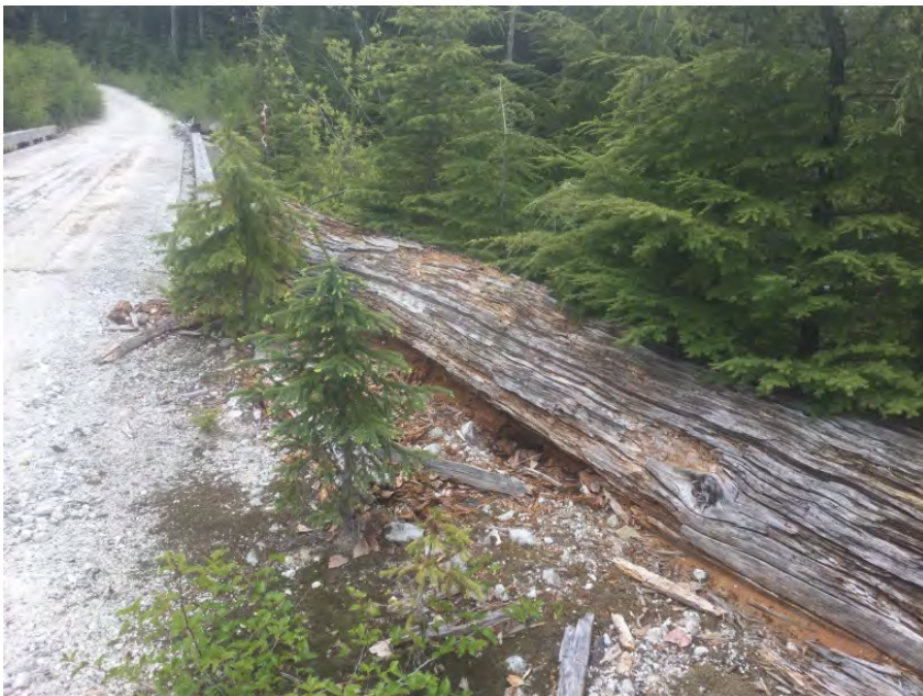
Typical fender log condition
